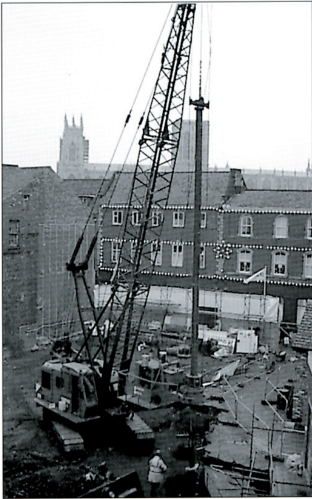
Mitigation Strategy in action: carefully positioned piling avoids excessive damage to important archaeological remains
