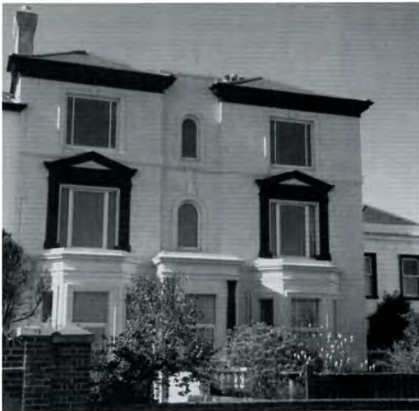
The use of article 4 Directions can be used to control the provision of appropriate windows in conservation areas. In this example the use of uPVC windows detract from the special character of this Victorian house (Deal)
