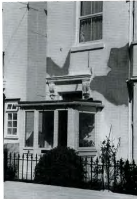
Inensitive alterations, such as the provision of this porch, can be controlled by the use of Article 4 Directions (Deal)
