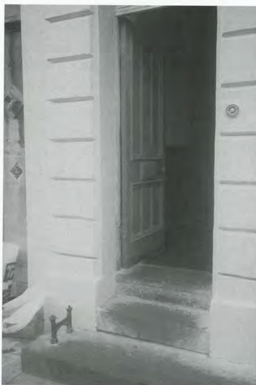
Section 215 notices can be used to deal with problems such as where important features have been left to deteriorate (Oxford)
