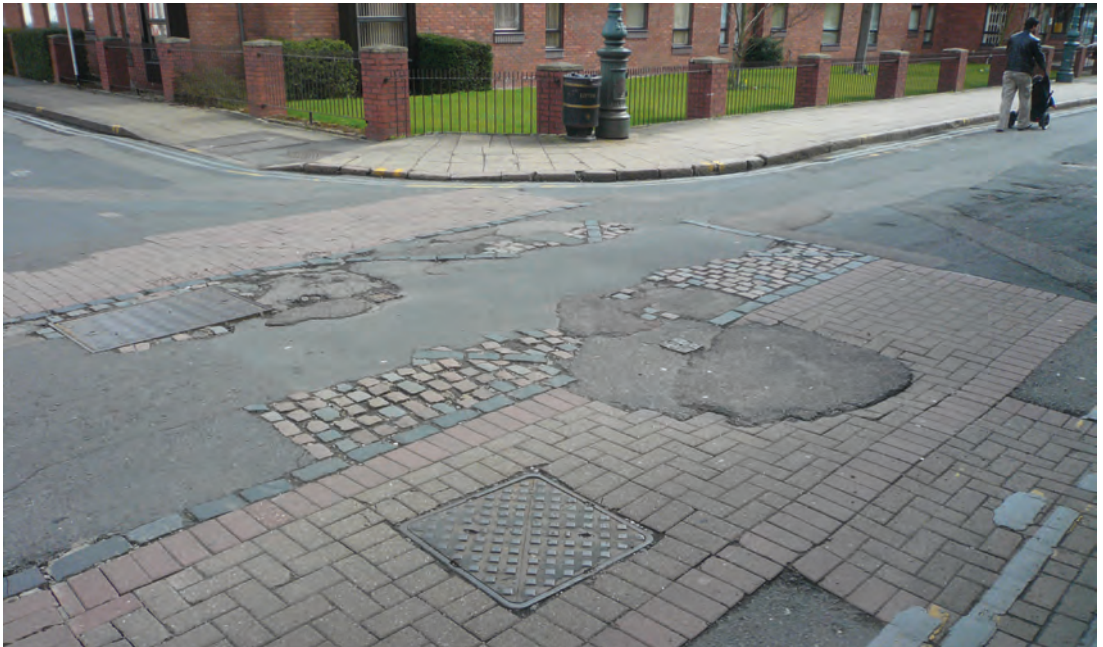
Figure 4: Neglected marker of former building; Hill Street Gate, Coventry: demolished late 18 th century, partially obscured by poor patch repairs over roadway marker of c. 1993.
