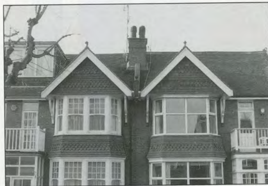
27. (above) Crude replacement windows.
