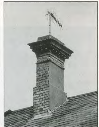
11. A fine chimney stack stripped of its character.
